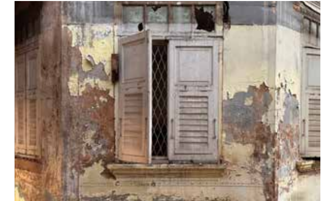
9. A Construction Site, Bangkok Demolition reveals the hidden beauty of a nearly century-old house, showcasing traces of past renovations and color transformations caused by chemical reactions.
